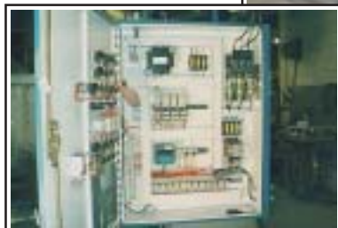
Left photo: Complete electrical controls system.
